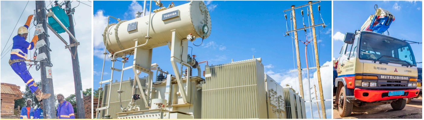
▲ UEDCL Technicians commissioning a transformer as part of the Company's strategic effort to stabilize power supply. The Company has increased the capacity of seven major substations across the Country to boost reliability
